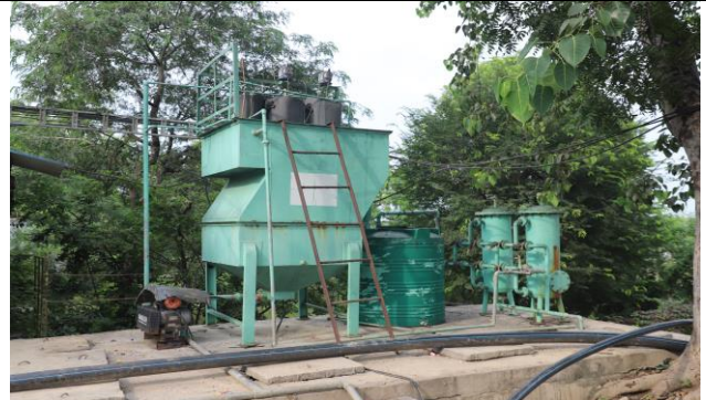
Effluent Treatment Plant
