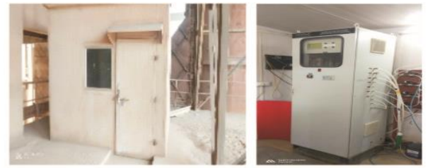
Continuous Emission Monitoring System
