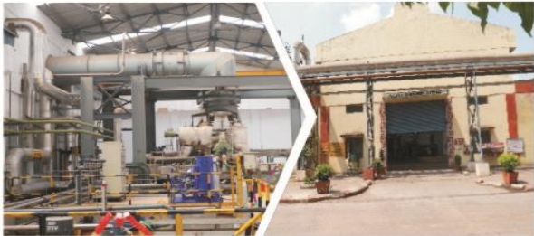
Waste Heat Recovery System
